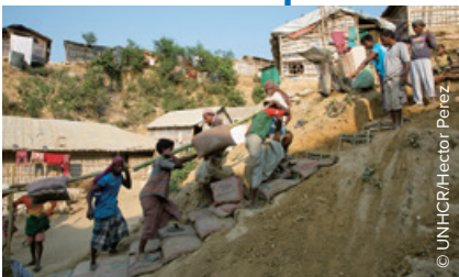
聯合國難民署與合作夥伴日以繼夜地建橋築路。UNHCR and its partners working around the clock to put in new roads and bridges.
