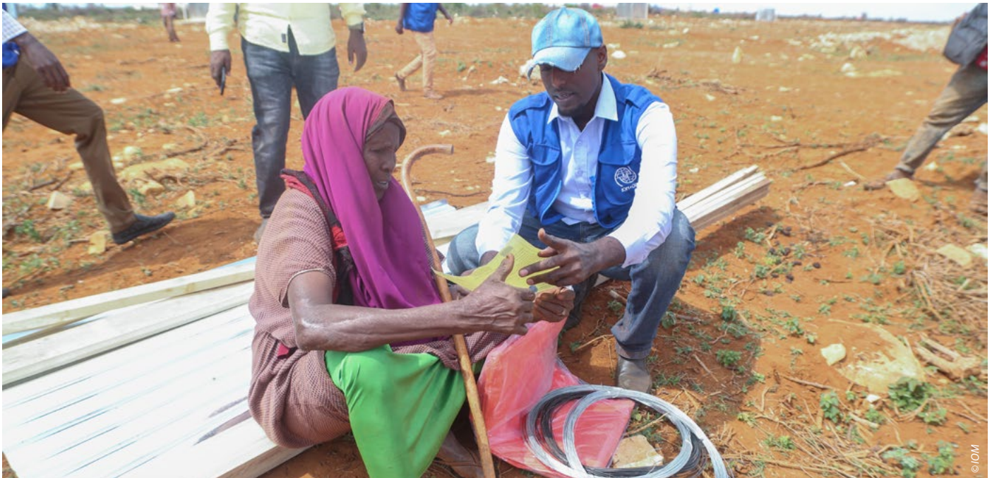
IOM staff from the Shelter and Non-Food Item (S-NFI) unit providing assistance on Shelter construction, Somalia 2019
