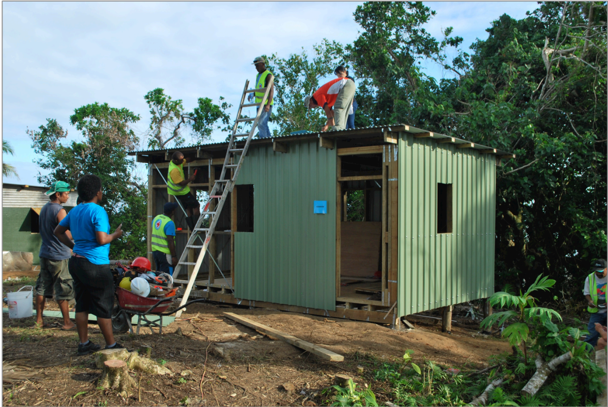
Building Back Safer technical training run in May by Shelter Cluster and Habitat for Humanity (Source, Shelter Cluster)
