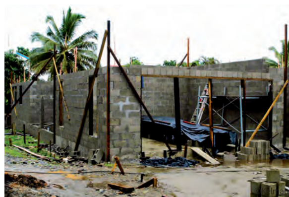
Poor quality cement block masonry house with steel rods
