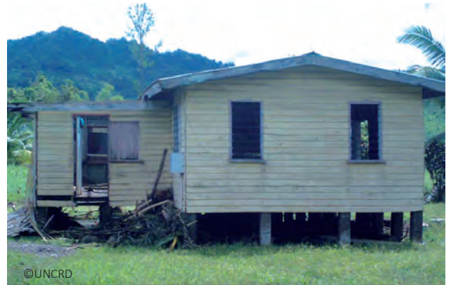
Transitional wooden housing: partial damage after 2016 cyclone Winston
