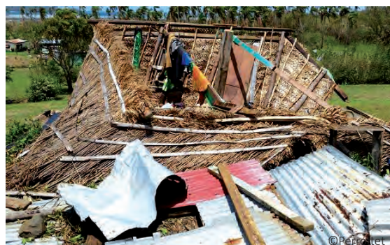
Construction with mixed materials: even if heavily affected, its lightweight limits risks of serious injury
