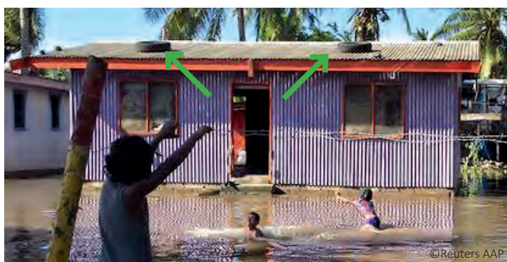
Tyres placed on CI sheet roof to reduce vulnerability to wind
