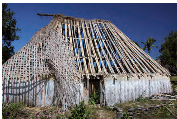
House damaged by a cyclone: a large quantity of materials can be reused for repair the existing house or to build a new one
