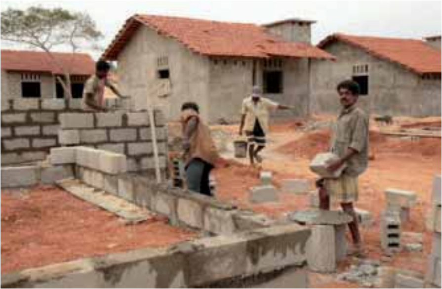
Men at work on houses built through the Community Recovery and Reconstruction Partnership (CRRP) in Trincomalee, Sri Lanka, 2007. Japanese Media Team
