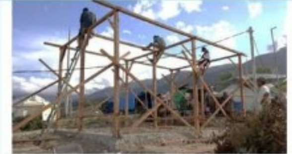
Project workers shall be minimal, i.e., not more than five individuals (or as per national guidance). Use preventive equipment.
