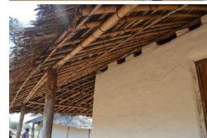
House in Mpale, Mangochi (top), House in Dzipsulle, Ntcheu (bottom). These two houses have a contact surface between the wall and the roof structure which is minimised using only some bricks to sustain the framework. This permits ventilation, but also allows for a better visual detection of termites paths and thus a better control of their attacks. © Jon Twingi
