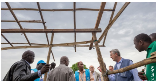
The UNHCR High commissioner's visit to Bentiu in June 2017 engaging UNHCR staff and the local authorities near a shelter under construction.
