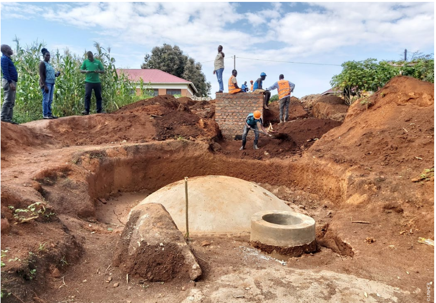
Biogas plant construction in a school in Kyangwali to reduce firewood use for cooking
