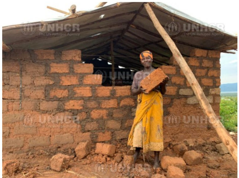
A Burundian refugee proudly shows the progress she has made in building her own house, using UNHCR's cash-for-shelter assistance in Mulongwe settlement, South Kivu Province. © UNHCR/Sanne Biesmans
