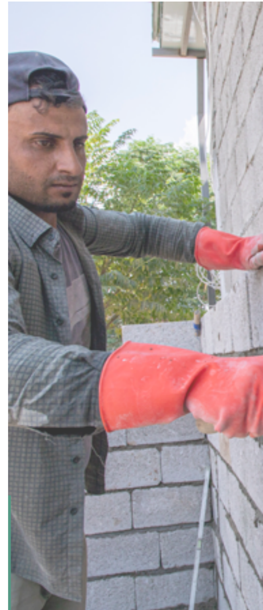
A total of 672 shelters in camps in Erbil Governorate got upgraded even though delay of infrastructure works were encountered. Infrastructure programs will put more focus on promoting self-reliance through community mobilization, improvement of social-economic conditions, social cohesion and accessibility, capacity building, and expansion of service facilities during the second half of 2020.
