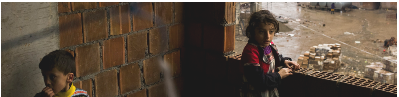
Two young IDPs stand at a damaged balcony in a building in Daben city, a housing estate with five buildings. Residents face multiple dangers including the cold, falling from floors or staircases or being hit by debris. There are 1.4 million IDPs in Iraq since January 2014, as well as 4.7 million returnees as of 30 June 2020. Photo by UNHCR / D. Nahr
