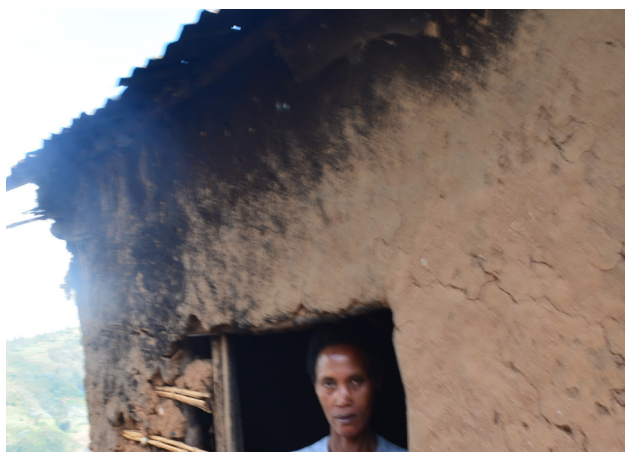
A portion of the house of MUKANDUTIYE Mwitigure close to the door, which seriously caught fire (photo Yves M.)
