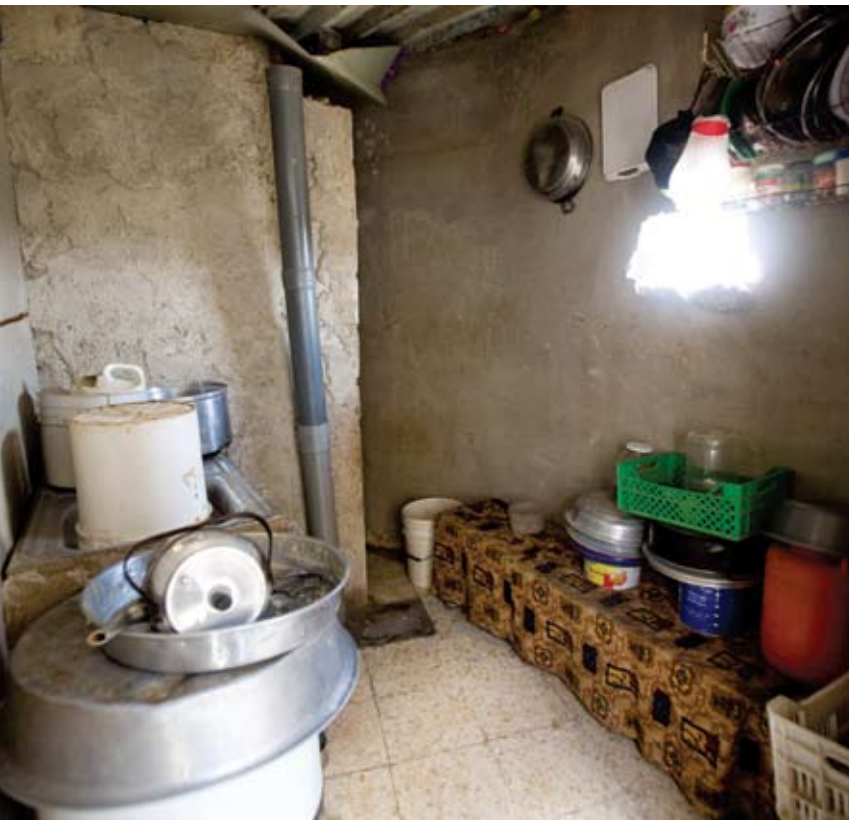
A shared cooking facility in Mufraq has a hole punched in the wall for a window. More than half of households have poor or worse sanitation.
