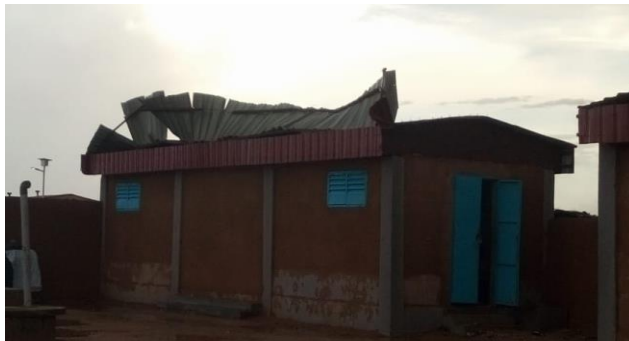
Damages occurred in the Humanitarian Center due to harsh wind and rainy storms during the last month/ APBE
