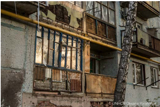
Shellfire-damaged windows in a building located in Svitlodarsk, Donetsk, Ukraine.
