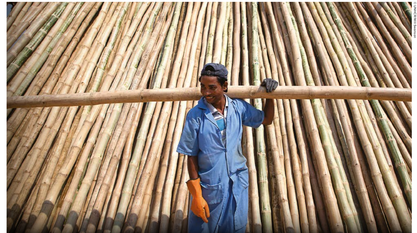
Nor Kalam, 25, helps to prepare bamboo logs for chemical treatment at Kutupalong camp, Bangladesh. Bamboo treatment brings more sustainable housing to camps.
