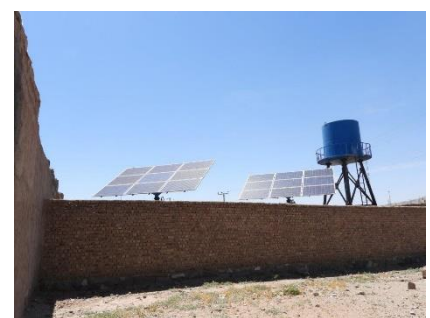
UNHCR's community-based protection programme constructs wells powered by solar pumps to provide safe drinking water to returnee and host communities. © UNHCR/D.Corcoran
