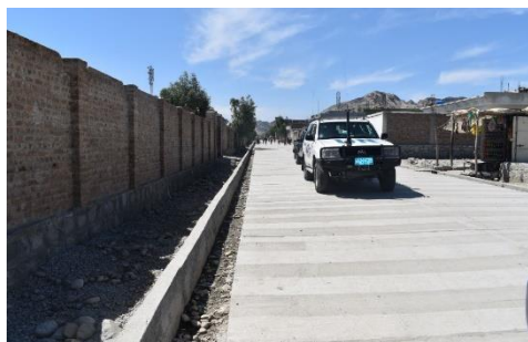
UNHCR encourages other partners to engage in projects to support returnees and host communities. UN-Habitat constructed this road in Daman. © UNHCR
