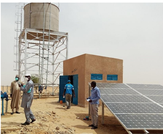
A hybrid water pumping station built in Assaga. More than 16,000 Nigerien and refugees have access to drinking water thanks to 5 water fountains powered by 28 solar panels and 1 generator.
