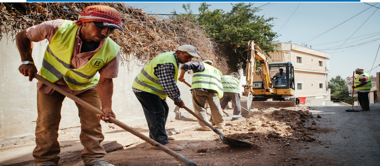
Workmen fill a ditch housing a water supply system being constructed by UNHCR thanks to European Union funding. A total of nine water supply and storage systems will be built through this support in the Bekaa Valley and North Lebanon ©UNHCR/M. Dudek
