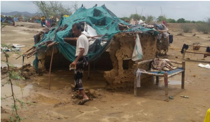
IDPs shelters damaged by the recent flooding in Abs district, Hajjah Governorate. Photo : Al-Amal Association | August 2016.
