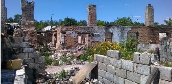
Figure 1-Category 4 damaged homes along contact where vulnerable and elderly still reside as they have no other housing solutions. Credit: A. Meyer
