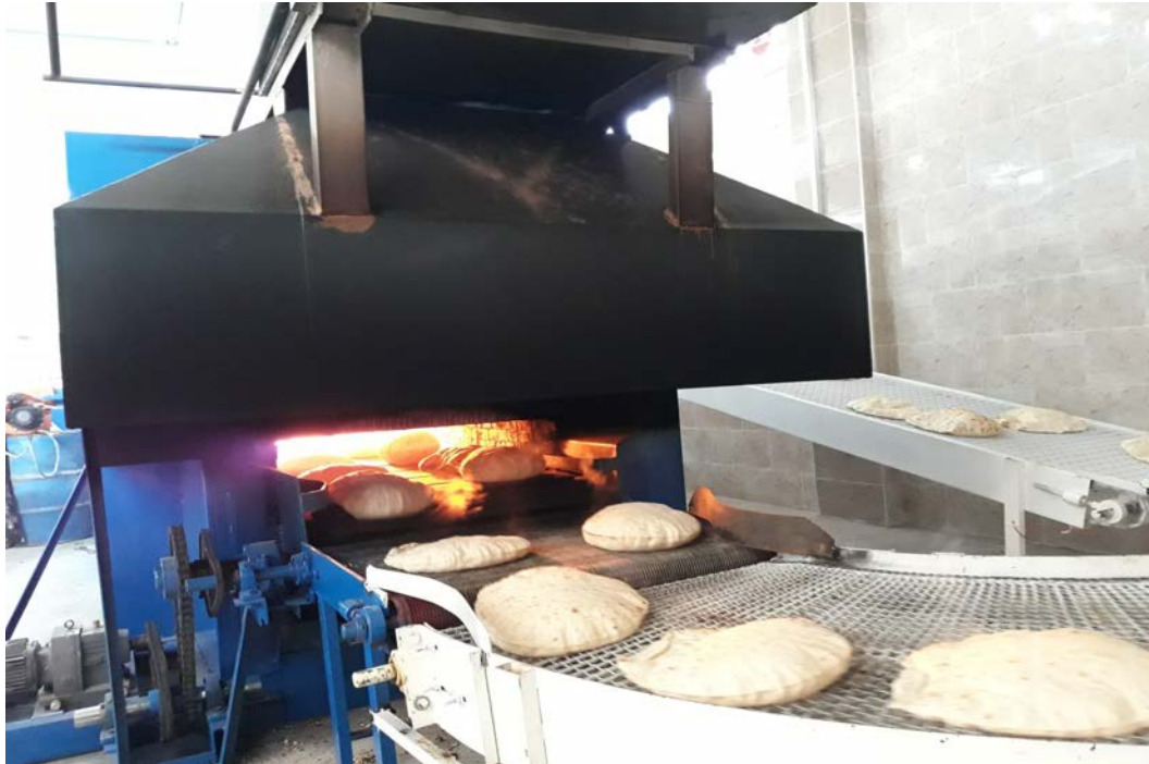
UNHCR in partnership with SIF installed a bakery production line. The bakery will cover 44,000 individuals with bread in 22 villages.
