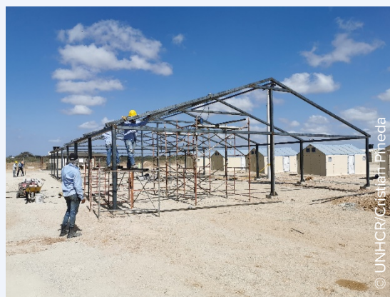
Staff building protector zones in the integrated assistance centre in Maicao, Colombia. The structure, when completed, will serve as a protective facility for children of Venezuelan refugees staying in the camp.
