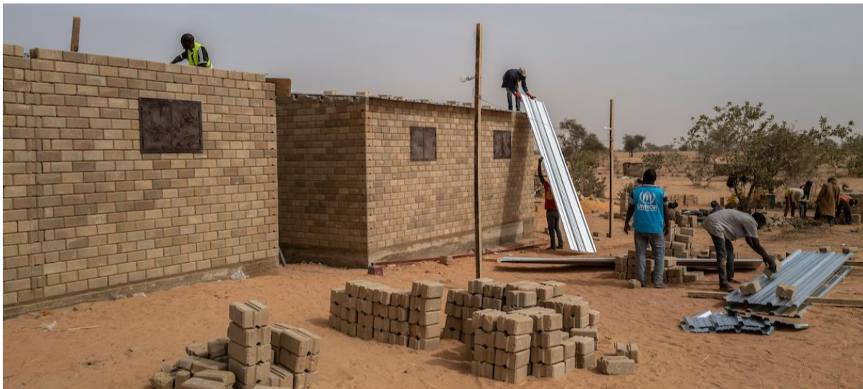
Construction of social housing for the most vulnerable refugee and host households is ongoing in the Tillabery region. UNHCR has pledged to construct 4000 social houses in Tillabery © UNHCR / Marlies Cardoen
