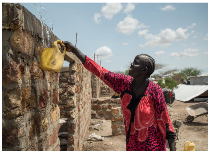
A refugee woman in Kalobeyei settlement pours water on her house to cure the cement. UNHCR has rolled out the first cycle of CBI for shelter in which 200 refugee families have started the construction of their permanent homes. UNHCR/Samuel Otieno
