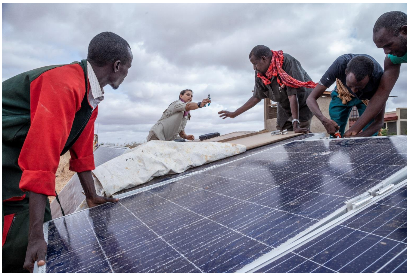
In Ethiopia, refugees and host community members use their training from Engineers Without Borders to maintain solar panels acquired with the assistance of the IKEA Foundation. © UNHCR / Diana Diaz
