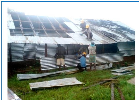
Shelter repair and maintenance at zone 0, Menik Farm IDP Camp, Photo Credit: UNOPS©
