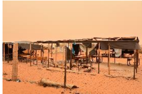
Schools in Mbera camp badly damaged by the sand storm. © UNHCR/José Manuel Cáceres
