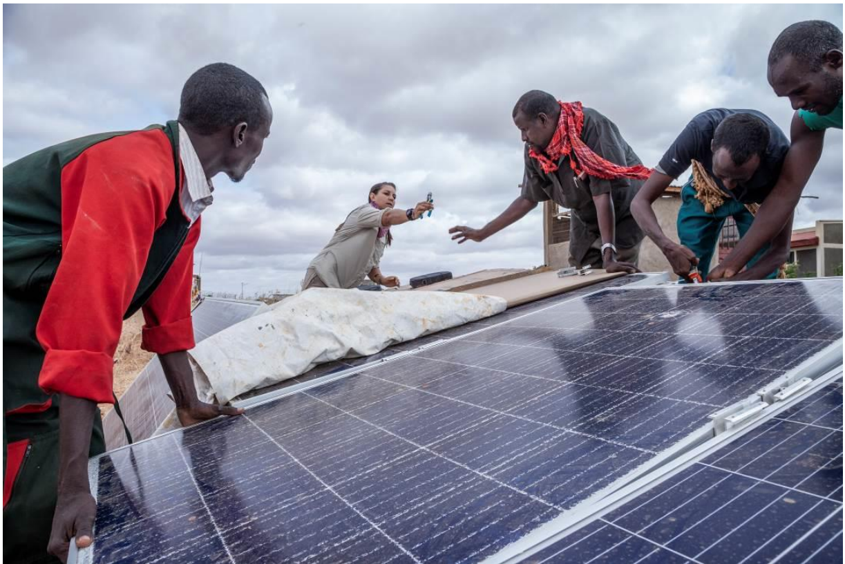
Refugee and host community-trained technicians maintain a solar panel that was broken. ©UNHCR/Diana Diaz
