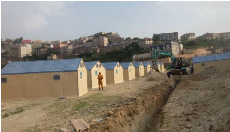
Refugee Housing Units (RHU) being installed by UNHCR through Jeel Albena Association for Humanitarian and Development (JAAHD) in Hajjah City. © UNHCR/JAAHD
