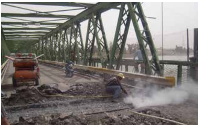
Maintenance work of the old bridge of Mosul, 2016 © UN-Habitat / Iraqi Urban Observatory
