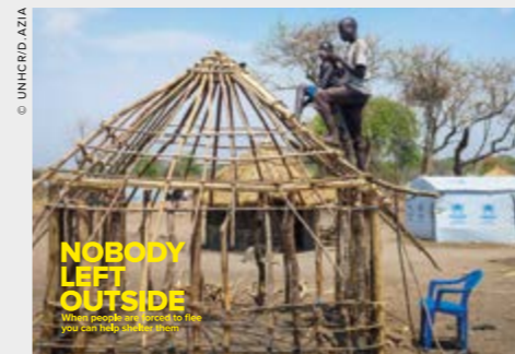
South Sudanese refugees Samuel, 16 years old, displaced from Lainya, and James, 17 years old, displaced from Wonduruba, work on the thatched roof of a tukul shelter in Bidibidi refugee settlement, Yumbe District, northern Uganda.
