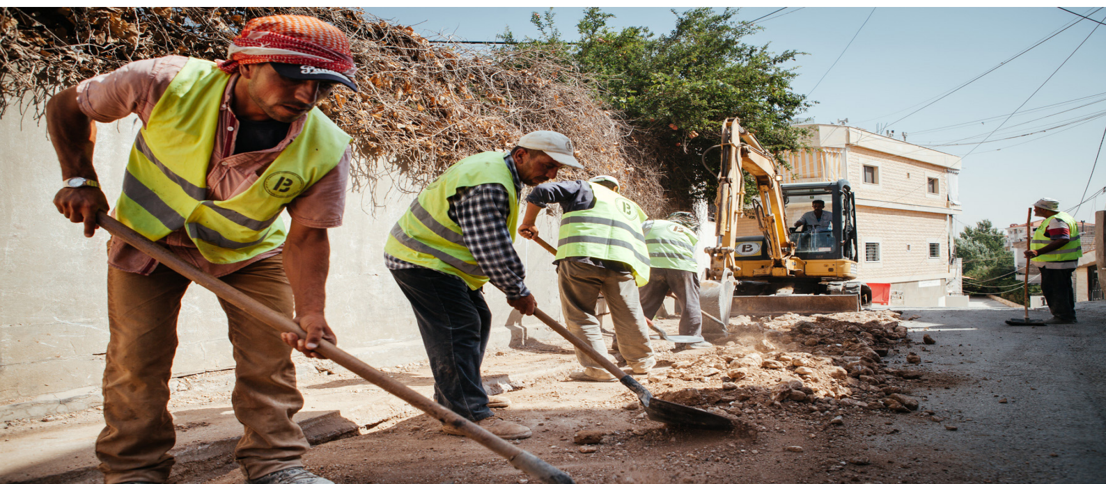
Workmen fill in a ditch housing a water supply system being constructed by UNHCR thanks to European Union funding. A total of nine water supply and storage systems will be built through this support in the Bekaa Valley and North Lebanon ©UNHCR/M. Dudek
