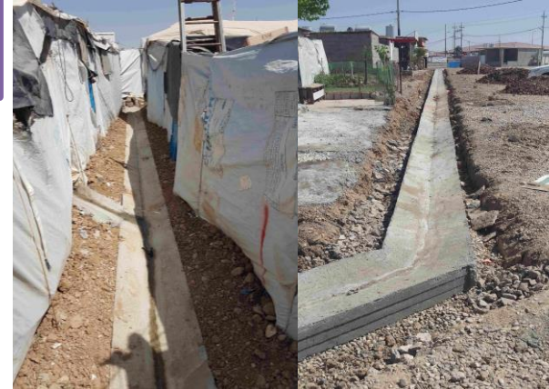
Construction of new open drainage channels behind shelters and along roadsides in Domiz 1 camp, Dahuk. UNHCR/Iraq/2016
