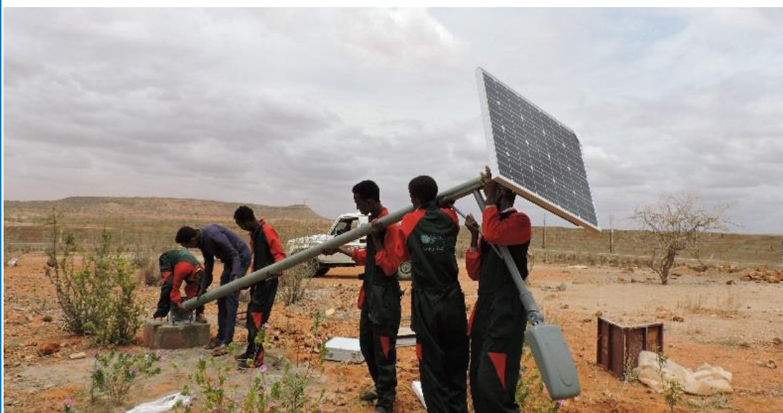
Installation of SSLs in Melkadida by refugee solar technicians @UNHCR Jeny Pathak
