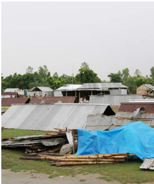
Household damaged by storm
