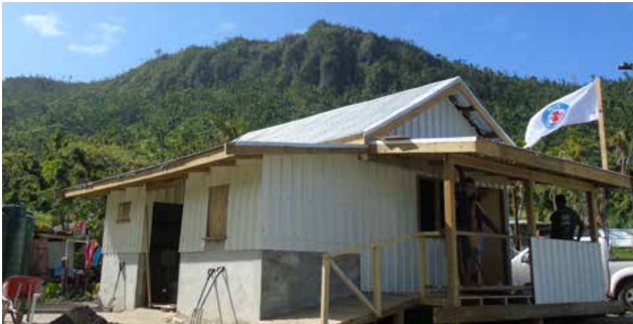
This house was built after TC Winston with Build Back Safer principles. (Source Fiji Red Cross Society/IFRC).
