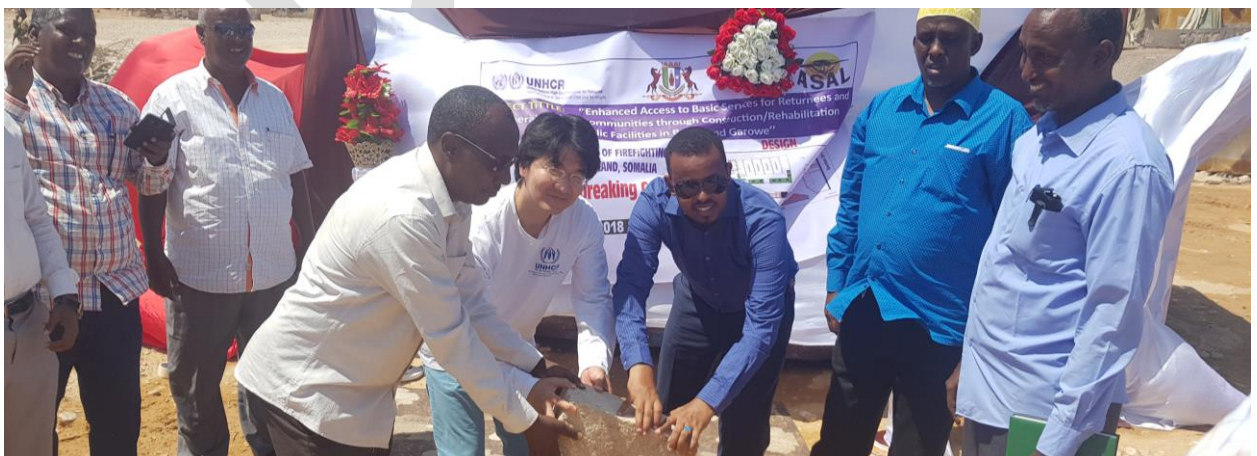
UNHCR with partners laid the foundation stone for a fire station. © UNHCR/April 2018
