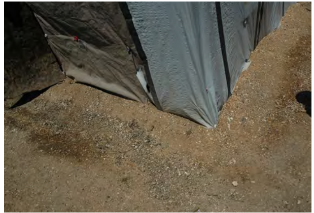
Base of shelter anchored with sand and soil. Drainage fall constructed to divert site water away from the shelter.
