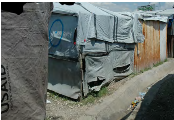
Poor quality plastic, poorly fixed and degraded. The shelter was slashed after the occupants had abandoned it.
