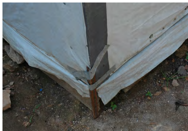
Steel peg to anchor shelter to ground, secured with hurricane straps. Pegs were relatively expensive and considered less priority by residents.
