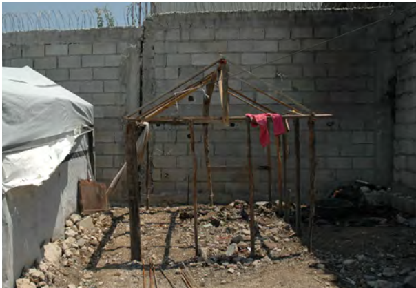
Small new shelter under construction, showing a greater constraint in availability and quality of framing materials, limiting shelter area, height and strength.
