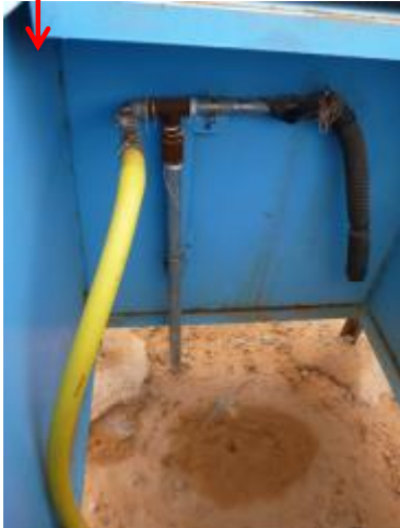
Detail of the communal tap from inside the box
