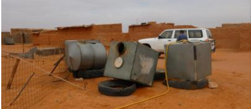
The right tank is being refilled (note the yellow flexible pipe)
