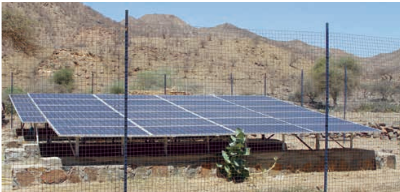
Climate change adaptation project installed solar energy to pump water for irrigating farmlands in Habero © UNDP/Mwaniki
