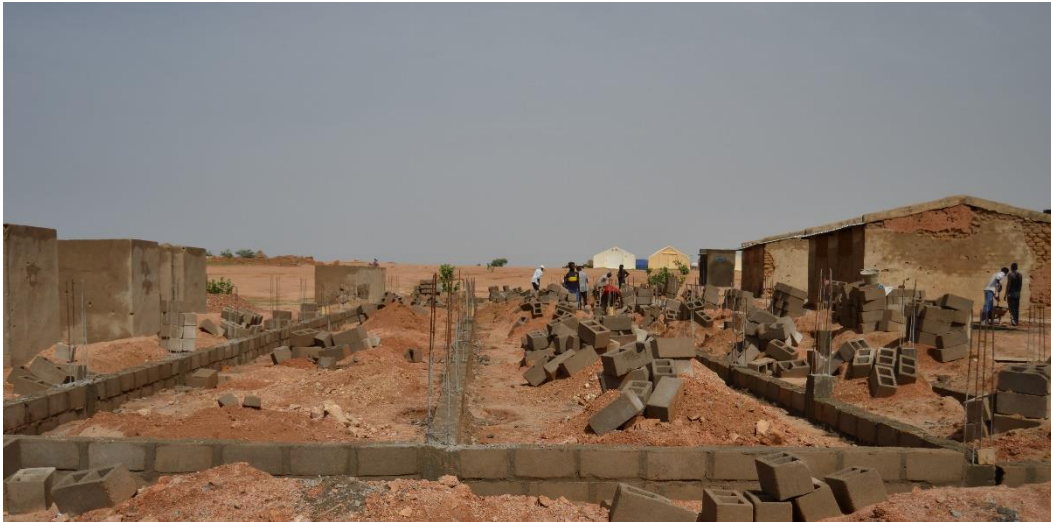
Some of the new classrooms being built (centre) and deteriorating ones (right) in the camp of Iridimi. Photo UNHCR/I. Diane
