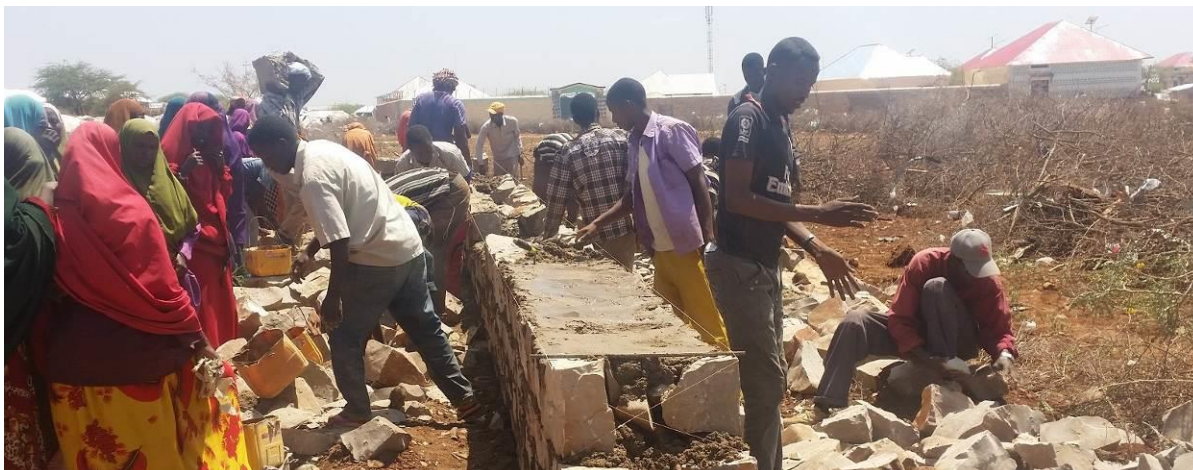
Community-based coexistence project through rehabilitation of a perimeter wall of the Halwadaag health centre perimeter wall rehabilitation. © UNHCR/Baidoa, 2017
