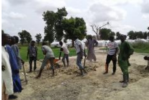
Community mobilization for sand collection to fill the potholes in the camp
