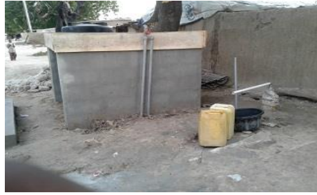
ACF water project in Damasak Shetimari
