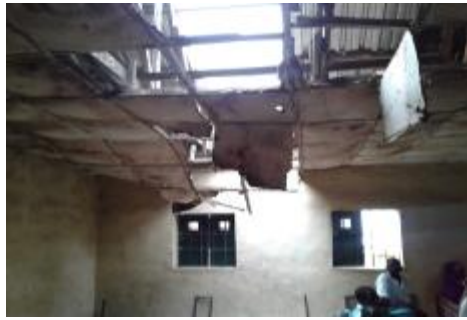
Destroyed classroom roof in Kuya primary school
