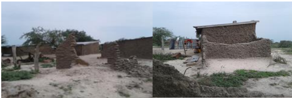
Houses destroyed by rain and wind
