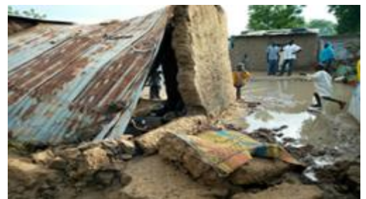
IDPs accommodation destroyed by rain
