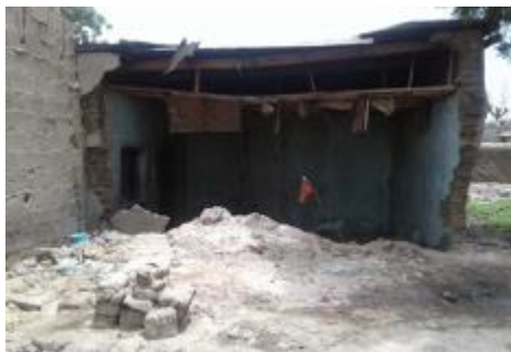
Most of their houses are destroyed by Boko Haram.
