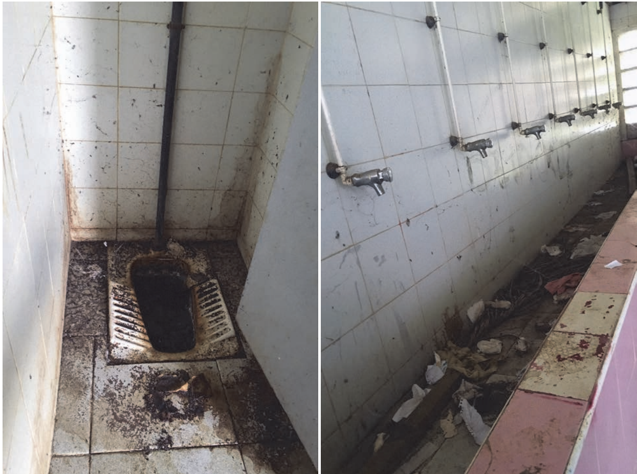
A bathroom at the high school, where there is no running water. ©2016 Human Rights Watch
