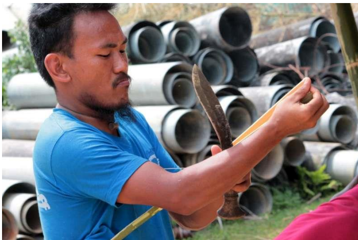
Sancha Hang Subba, a refugee from Bhutan, cuts bamboo with a Khuluri whilst constructing a temporary shelter for earthquake affected families in Ramechhap district in Central Nepal. Subba is leading a 14 member refuge construction team supporting the local community. ©UNHCR/D.D.Shrestha
