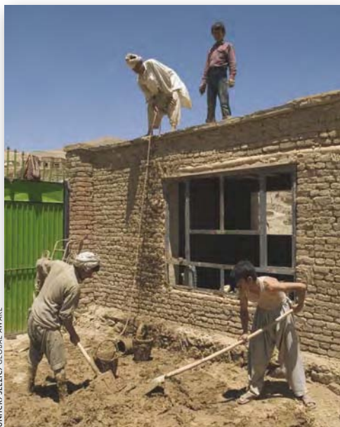
UNHCR works with its partners in providing building materials for a housing programme for Afghan returnees.
