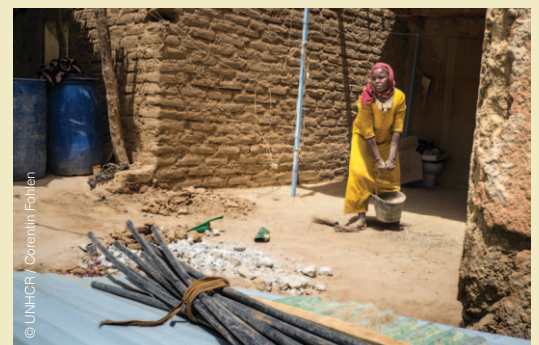
Aza does construction work. It is the only way she can earn enough income to feed her family.
