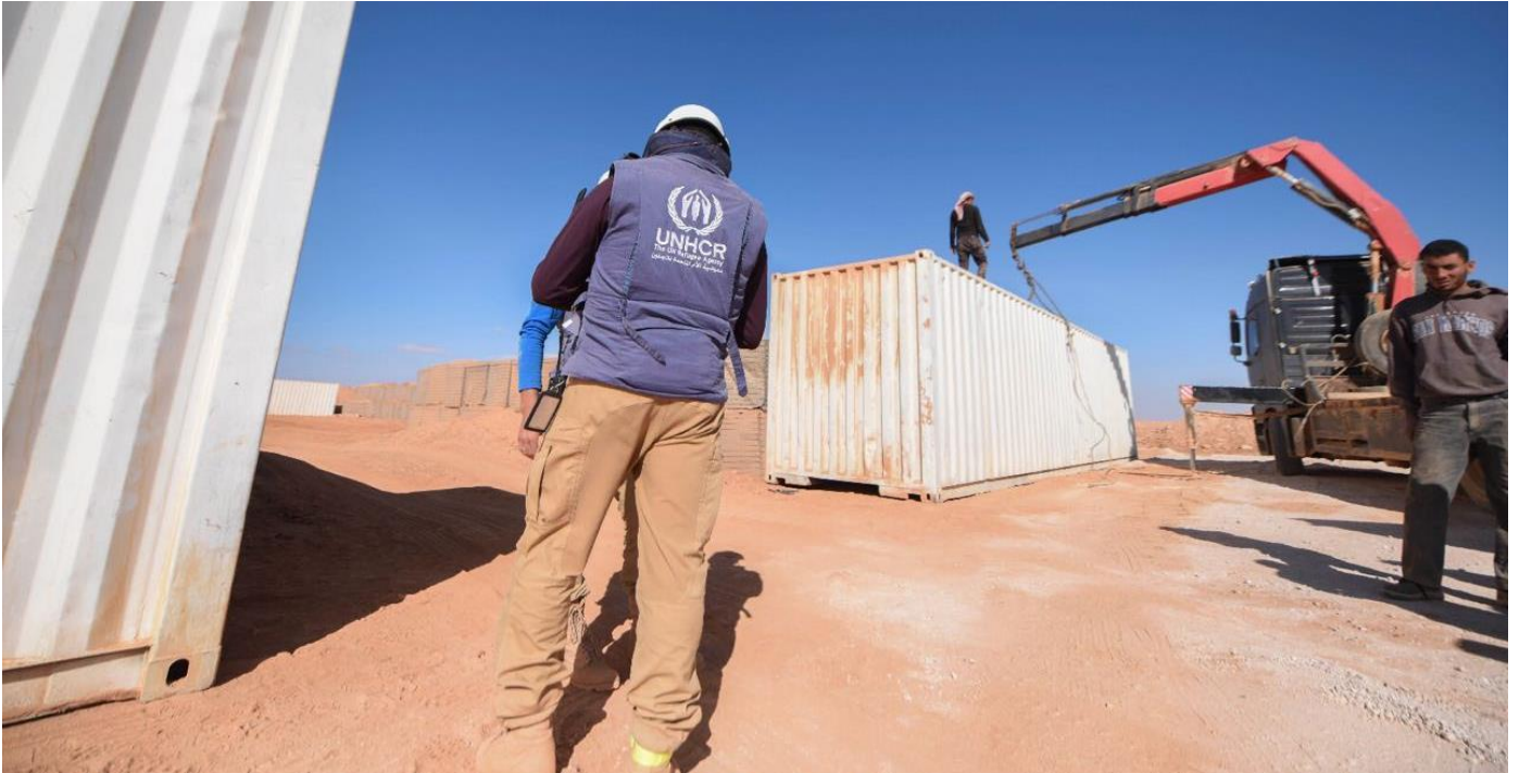
UNHCR field staff working near Rukban on the construction of a new service facility to support the provision of assistance to the area. ©UNHCR/Mohammad Hawari
