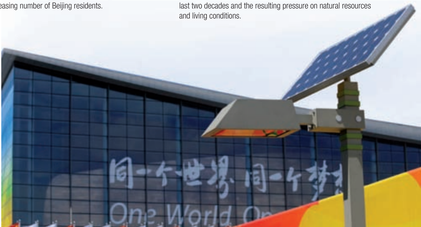
Solar-powered lighting in the Olympic Green.
